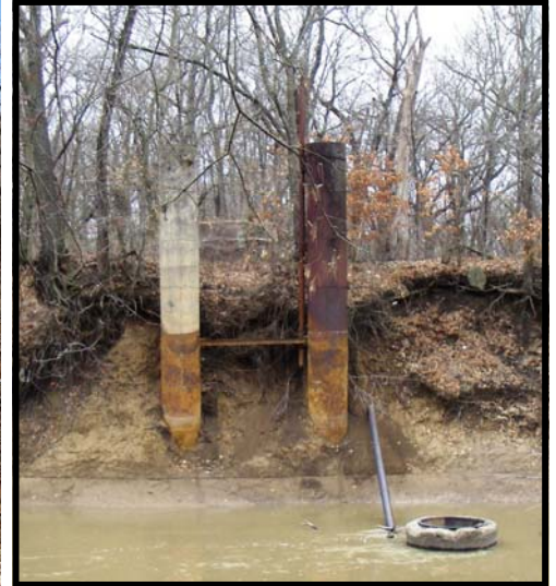
Traveling east from PSO the Interurban crossed a bridge. The support system for this bridge can be seen south of the Frank Phillips Blvd. Caney River bridge.
